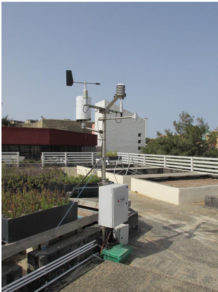
Figure 3 The weather station on the experimental green roof used - Malta
